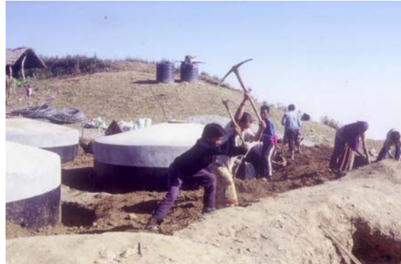
Namje villagers built a water supply system capable of pumping 12,000 liters of water per hour.
